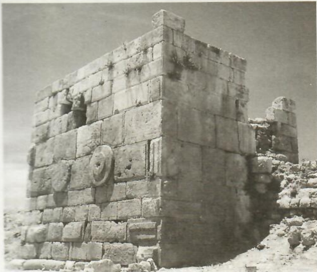
The south (left) and east (right) walls of the tower before restoration
